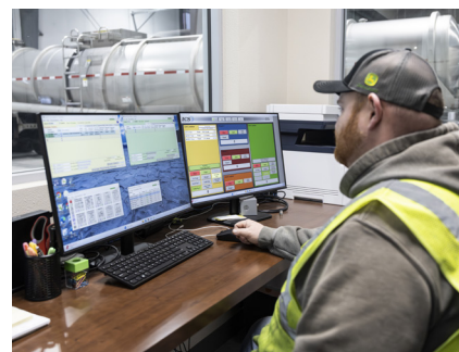
The new facility is fully automated with ICS ControlPro and ICS 480. ICS ControlPro manages customer tickets and batches, the 24-7 unattended loadout bay, and sending/receiving information from Nutrien's SAP software.
