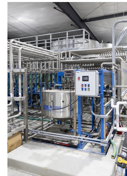
The site features MEI turnkey solutions such as this Premix Tank System.
