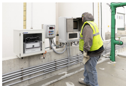
A third unattended loadout bay allows for round-the-clock customer service without additional staffing requirements.
