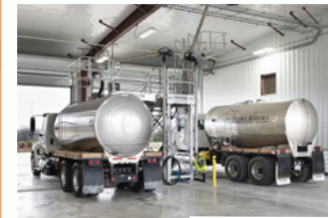
The liquid facility features two bottom and top load attended bays to increase throughput.
