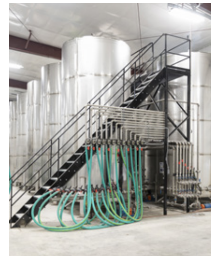
An automated tote repackaging area means the location can fill small totes in addition to large semi loads.
