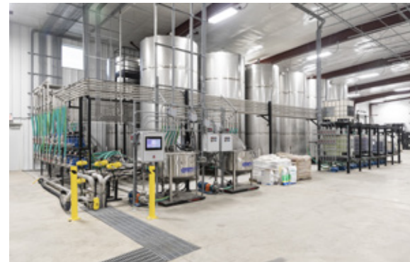
All the equipment, plumbing, metering, and controls were engineered by Murray Equipment. The goal was to help Conserv FS support the grower of the future.
