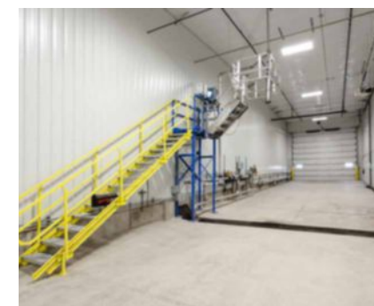
The Unattended Loadout bay allows customers and transport drivers to pick up loads 24/7.
