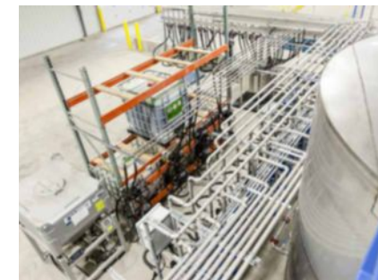
Murray Equipment also supplied the liquid handling equipment used in the facility.
