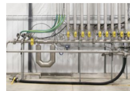
The facility features a third 24/7 unattended bay to allow trucks to pick up product and service customers round-the-clock.
