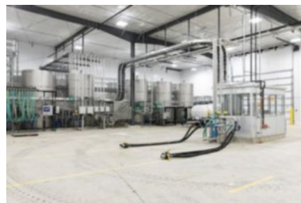
With the facility's 2 attended loading bays, vehicles and containers of various sizes can be filled quickly and precisely.
