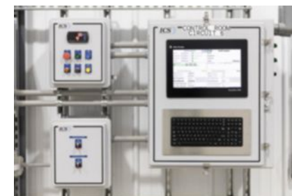
The same ICS ControlPro software that runs the facility, is used in the unattended bay control panel for seamless operation.
