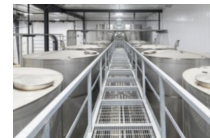
46,000 gallons of herbicides are stored inside in a series of stainless steel tanks.
