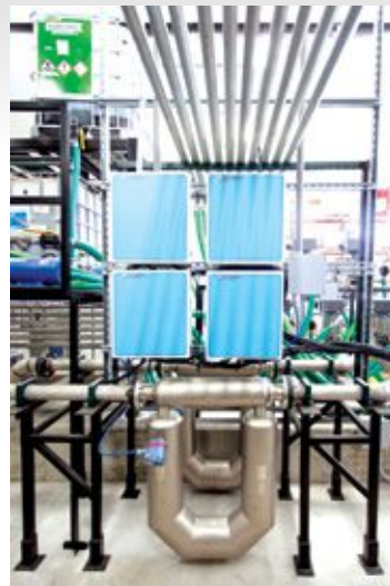
To achieve speed, the facility has two mass flow meters for filling two trucks at once. Murray Equipment supplied both the automation and the pumps, meters, hoses, and other equipment.
