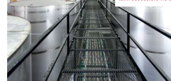
To store crop chemicals, Gateway FS installed 9 stainless steel tanks and 1 poly tank accessible via catwalk.
