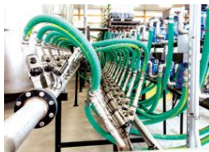
The facility incorporates 22 TCS 682 meters to produce precise hot loads and include hand-adds.
